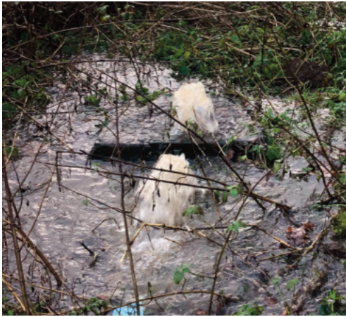
Leaking sewage pipe, Egton Estate
